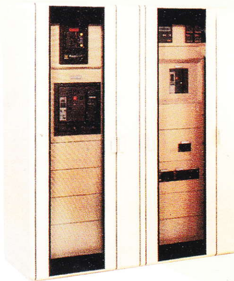
Distribution and protection panels
